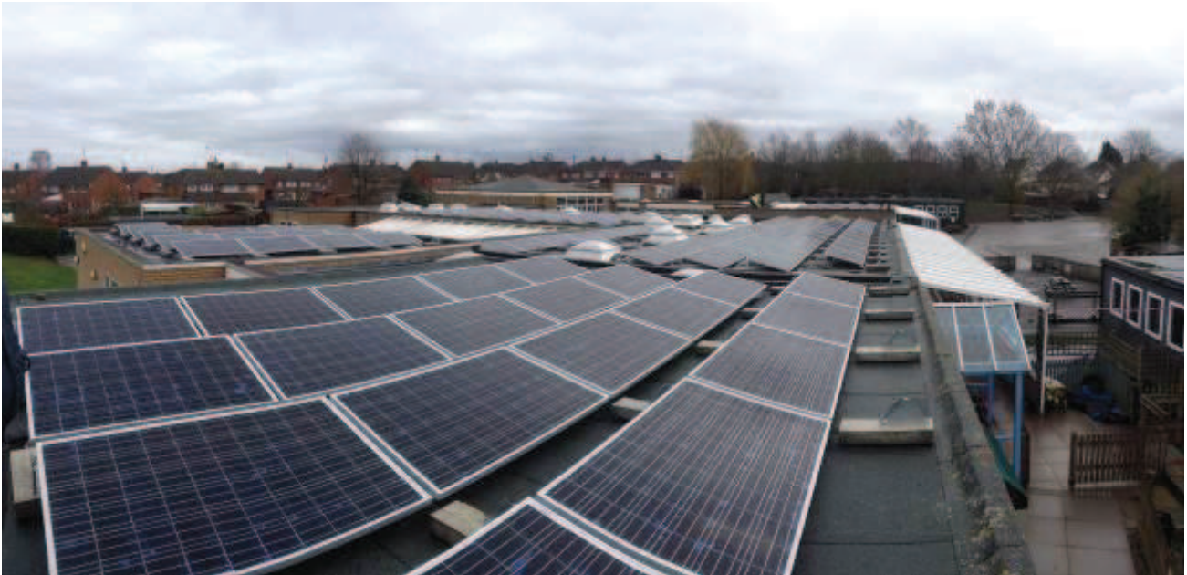
Figure 4: Solar Panels installed at Leedon Lower School
